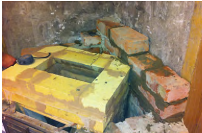
Figure 1.25. Continuing the laying of bricks at the rear. The gap between the fire wall and the rear masonry works as an insulator which keeps the warmth from transferring into the walls. It also allows the bricks to expand without breaking the stove.
