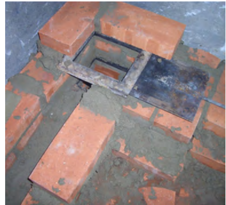
Figure 2.57. Tile row 3: the two dampers can be seen at the start of the chimney. To the left we have built the air duct for summer ventilation. (See also drawings.)
