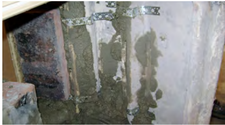
Figure 2.26. The cavity behind each tile is filled with thin bricks and clay mortar.
