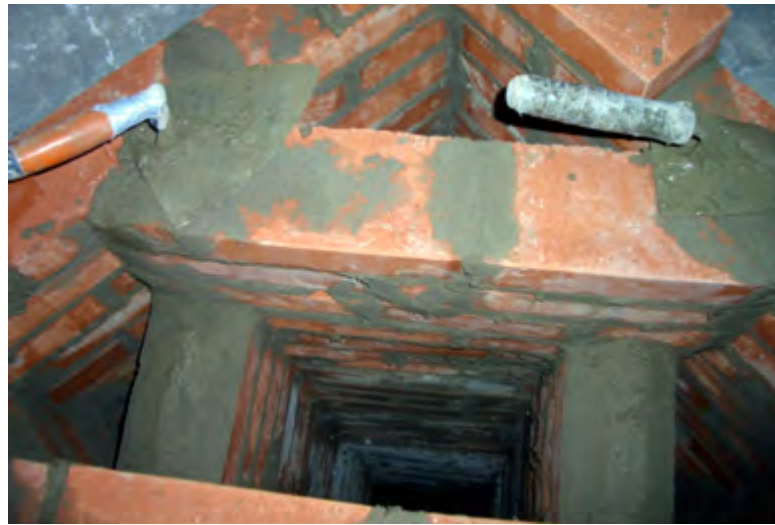
Figure 2.55. Looking down the system of flues just before the top was closed with solid brickwork.
