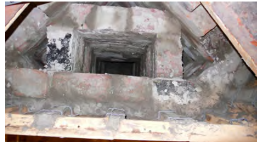
Figure 2.50. A view down the inside of the stove from the level of tile row 6.
