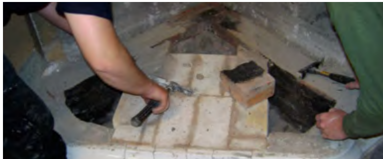
Figure 2.21. This is where we started the rebuilding of the stove. The bottom two rows of tiles were already in place (they were intact and therefore not dismantled). Before laying new bricks the base had to be cleaned and the old mortar removed.
