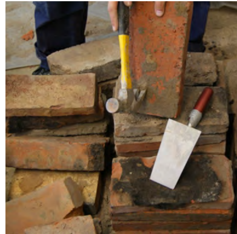
Figure 1.10. Cleaning the bricks is done by using a hammer and a trowel. Clay mortar comes off quite easily but the job is dusty and dirty.
