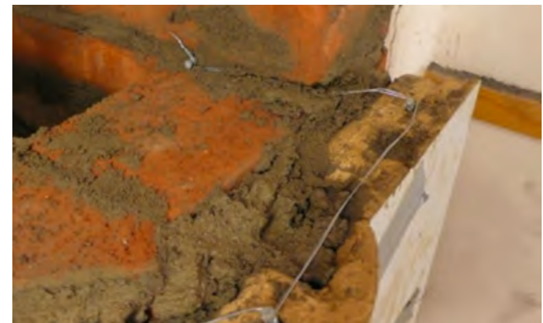
Figure 2.54. The wire is secured by a nail in the mortar joint of the side wall of the stove.
