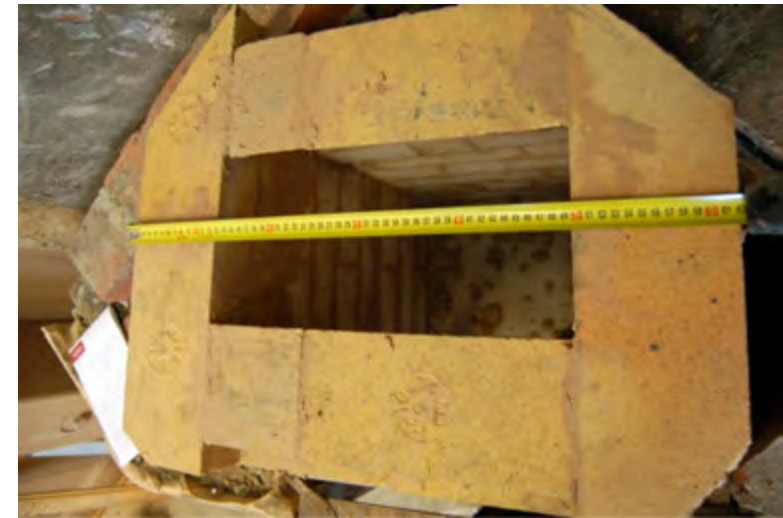
Figure 2.34. The middle flue is narrowed at the back and front of the furnace with a row of bricks that have been shaped with an angle grinder. This bottle neck will improve the draught in the flue.
