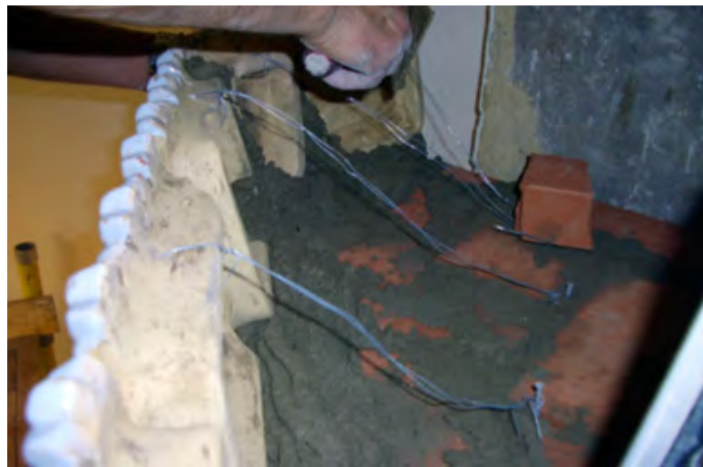
Figure 2.59. The masonry work for the stove is finished when these wires are finally covered with bricks and mortar.
