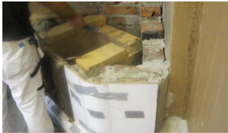
Figure 1.22. Laying the lower part of the furnace. Fireproof bricks and mortar were used. The masonry of the furnace should be bonded together with thin joints (1–2 mm) and separated from the rest of the masonry that has wider joints of clay mortar (13–15 mm).
