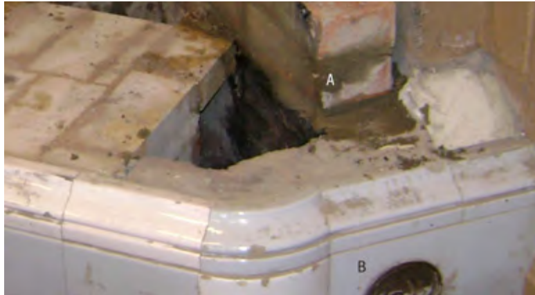
Figure 2.22. (A) The bricks are laid with clay mortar and with a 2 cm wide gap between the fire wall and the backside of the stove. (B) At the bottom of each side flue there is an opening with a metal cap. When the chimney (in the back corner of the stove) is swept the soot can be removed through these horizontal flues. The side cannels also join underneath the furnace floor and lead to the chimney in the back.
