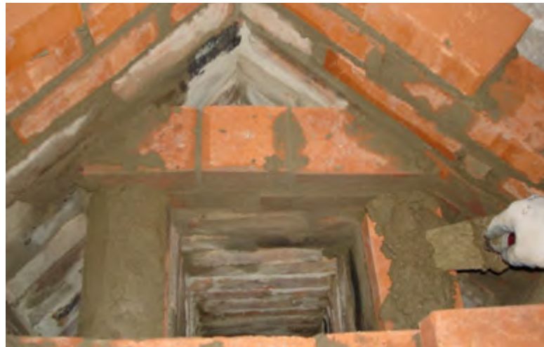
Figure 1.44. Day 5. Finishing the central flue just before installation of the last row of flat tiles. The tops of the side walls of the central flue are rounded to direct the air-flow to the flue pipes.
