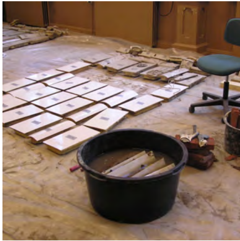
Figure 1.11. The tiles were soaked in water to soften the mortar. Three rows of the tiles on the floor have been cleaned and the lower rows of tiles are already assembled on the stove.
