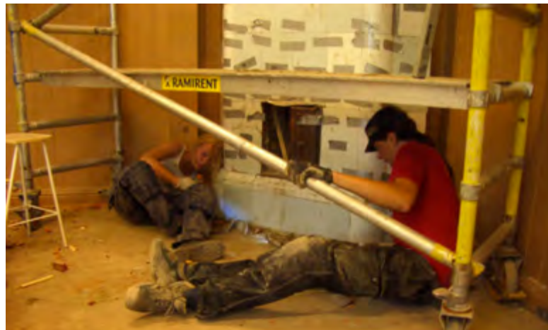
Figure 2.56. It is important to clean the bottom of the smoke flues from mortar droppings before the mortar sets!
