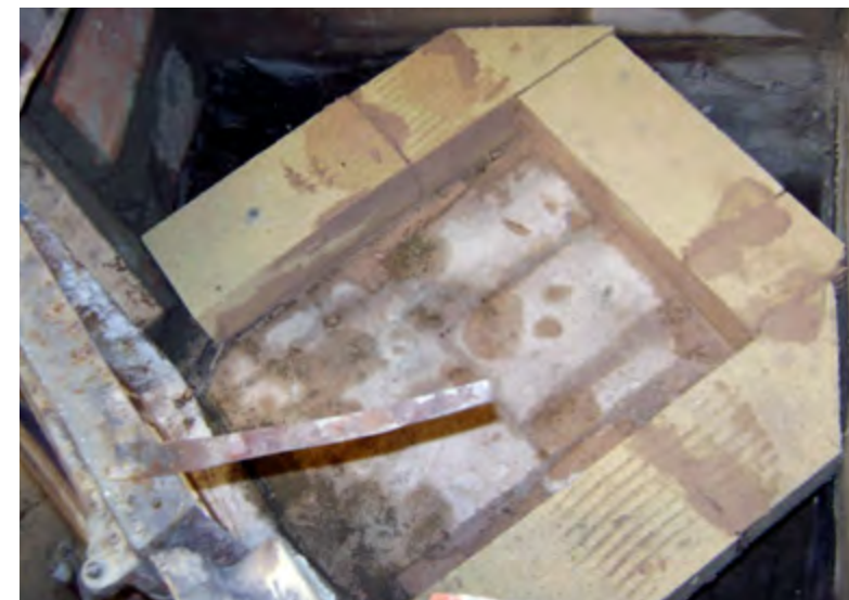
Figure 2.31. Metal straps connected to the cast iron frame are placed in the joints of the brickwork. The furnace is being constructed.
