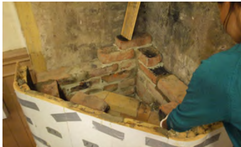
Figure 1.40. Five more rows of fire-proof bricks are layed up from the furnace. From then on the central flue is built using ordinary bricks and clay mortar.
