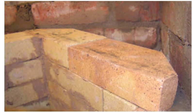
Figure 1.16. Fireproof bricks and mortar are used for the furnace. The bricks have to cover each cross-joint of the previous course.
