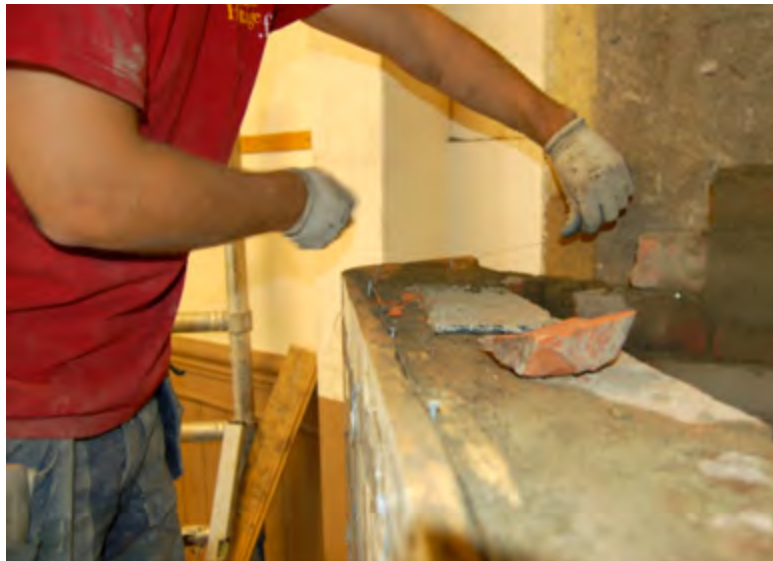
Figure 2.38. Nails are inserted into the existing holes in the flanges of each tile and tied together with a baling wire which is fastened in the joints of the rear brick course.
