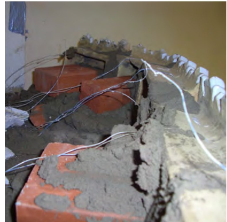
Figures 1.47–48. The chimney was repaired ( left ), before the crown tiles were finally inserted.
