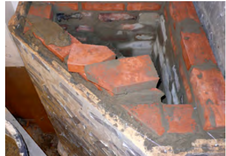
Figure 2.53. One and a half courses of the new bricks were laid. Before continuing the baling wire was attached as described before.
