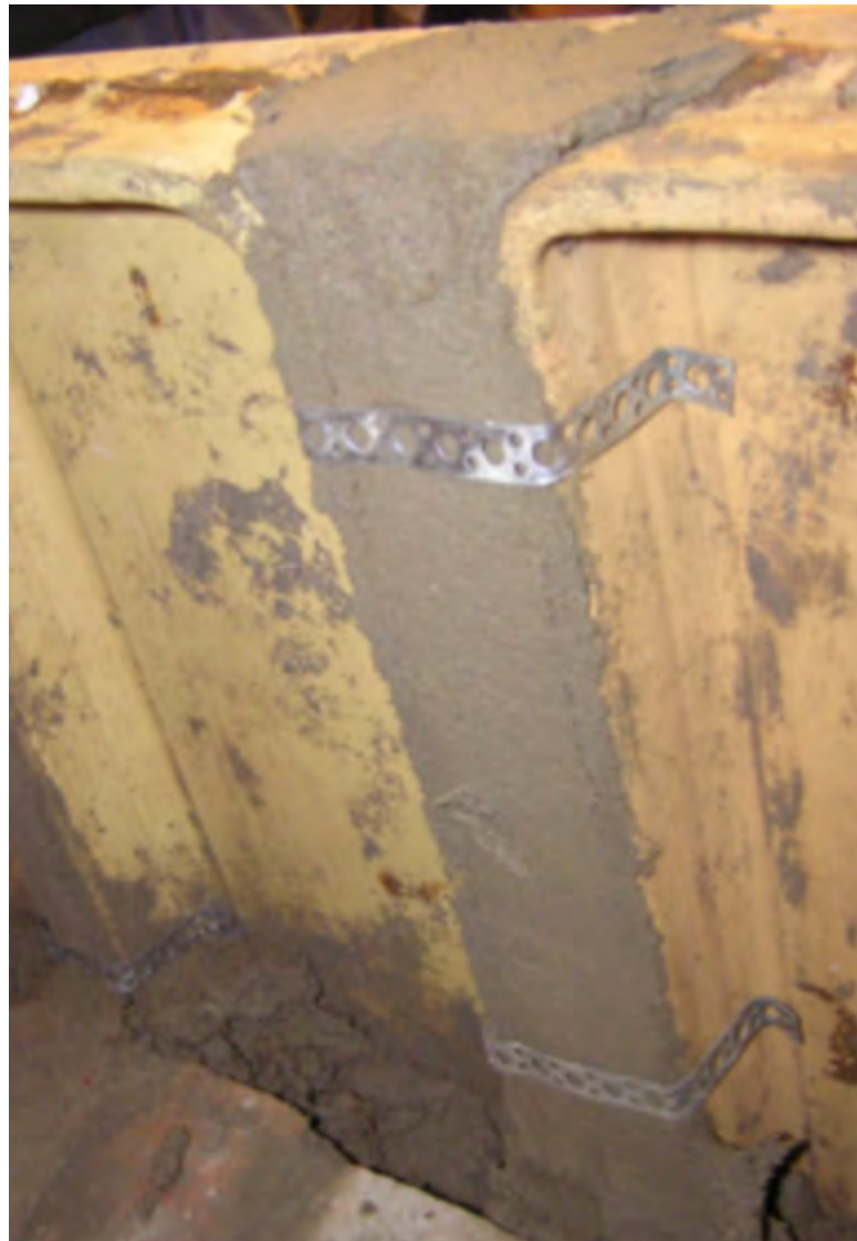
Figure 1.32–33. When the tiles are in place, the gap between them is filled with clay-mortar. Then two clamps made of perforated metal strap are bent to hold them together. The cavity on the backside of the tiles is then filled with mortar and thin bricks. Inside this a wall of bricks is built to finally stabilize the front.
