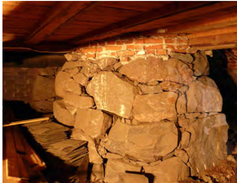
Figure 2.1. Every kind of stove or fireplace has to stand secure and immobile since movements in the masonry would lead to cracks and obvious fire hazard. This enormous dry laid foundation supports the stove whose dismantling and consequent rebuilding is described in the following. The stove itself weighs several tons.
