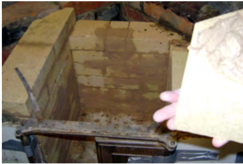
Figure 2.32. The fireproof bricks are built to the upper part of the cast iron frame of the shutters.
