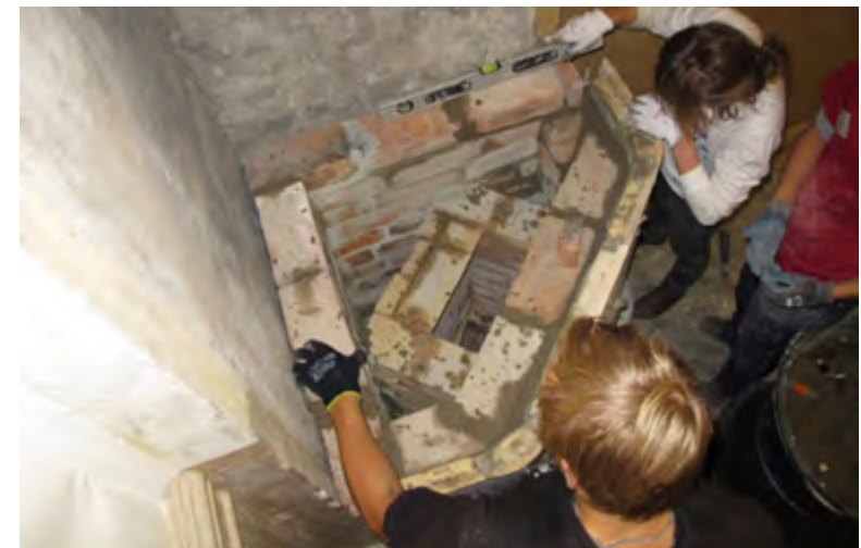
Figure 1.17. A spirit level should be used to level the bricks and help make the structure straight and secure.
