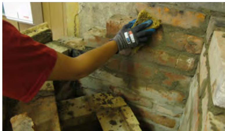
Figure 1.19. Washing off the clay mortar from the bricks in order to smoothen the walls of the flues.
