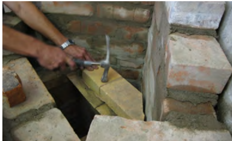
Figure 1.18. A hammer is used to adjust the bricks and tighten the joints.
