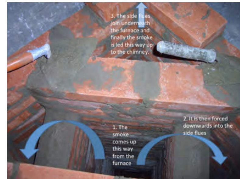
Figure 2.60. View down the flues at the level of tile row 4 (see also drawing). The next row of bricks will close the front flues.
