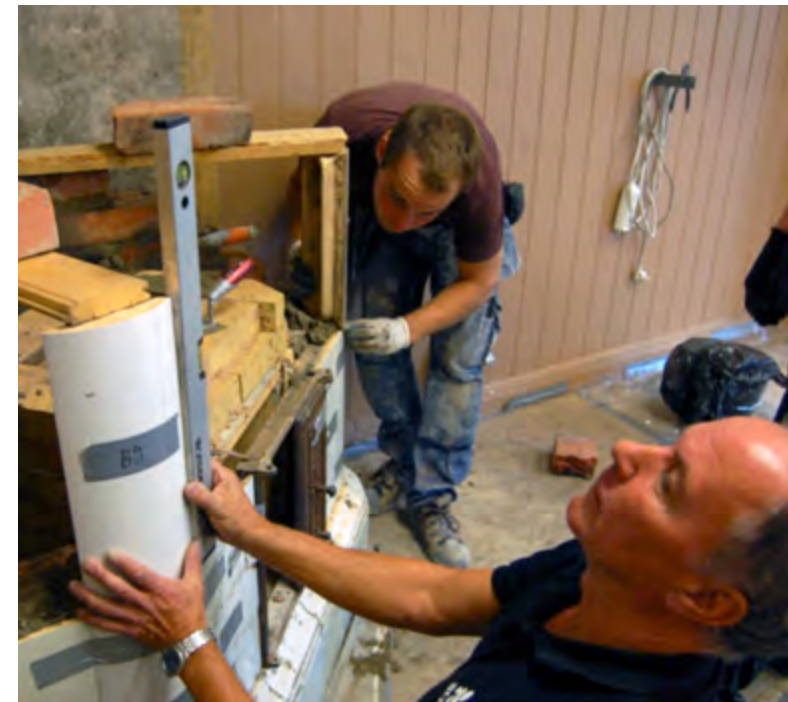
Figure 2.40. The corner tiles of tile row 9 are aligned with spirit levels. A small amount of mortar is placed beneath them before they are put in place. Master mason Krister Lindroos ( in the front ) assists with the difficult parts.
