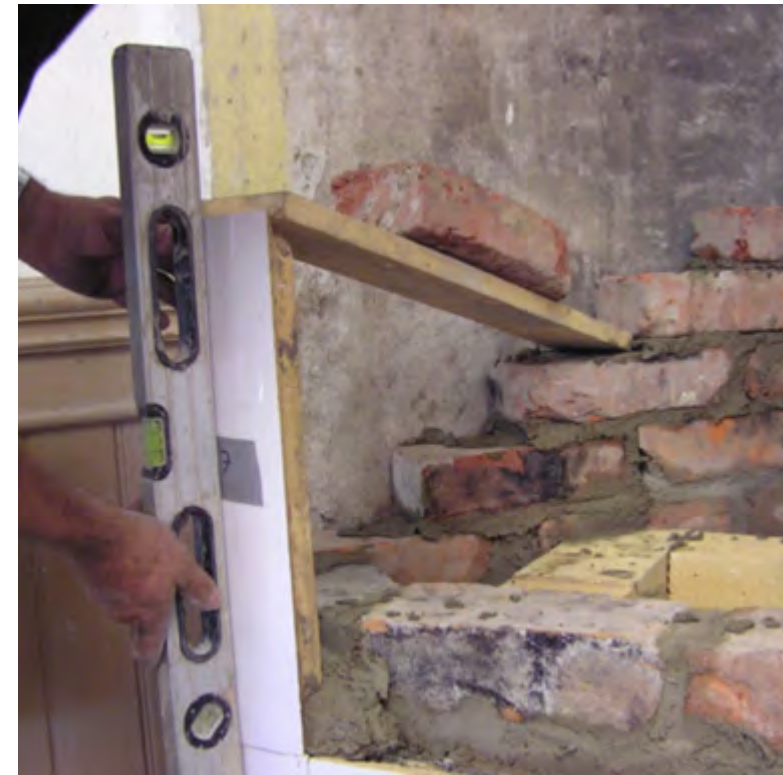
Figure 1.28. Corner tiles are the first to be installed. Therefore it is important to compare the distance between them with the width of the middle tiles. To keep the first tile in the right position and angle, it needs to be pressed downwards. A board with a weight is used. This is why the rear masonry needs to be built before the tiles are placed.
