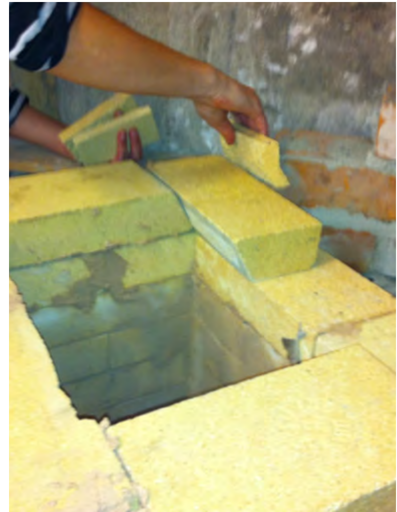
Figure 1.23. The rear masonry was laid to the height of half of the next tiles to be used as a support for the tiles.
