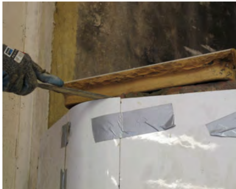
Figure 1.30. Correcting the size of the tiles can be done either by filing or using an electric saw.
