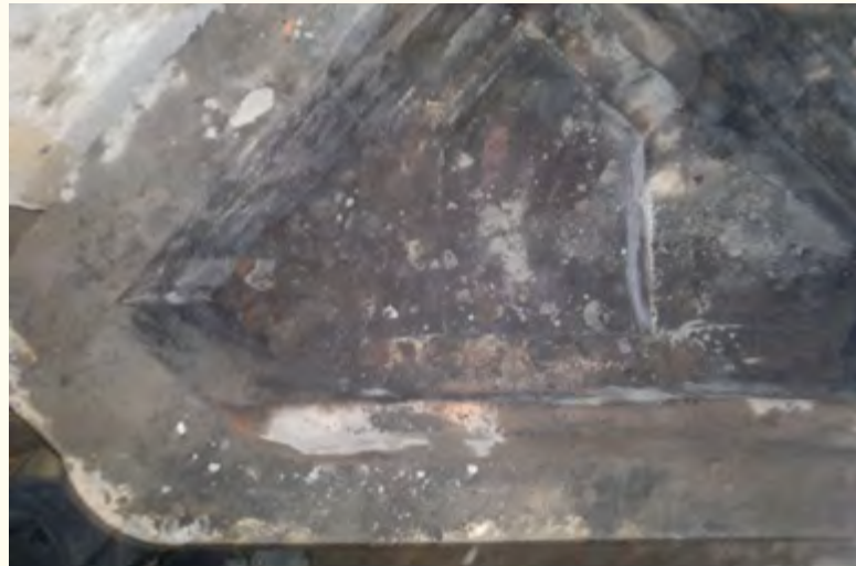
Figures 2.14 a, b. The ninth tile row is still in place but several rows of brick have been taken out from behind it. Here the floor of the furnace can be seen. This is where the dismantling was stopped because the bottom of the stove was intact and it was of course easier to start the rebuilding from a foundation that was of the correct size and shape. Above: measured drawing of the same.
