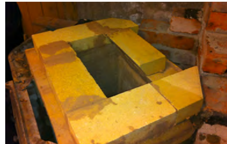
Figure 2.35. Side view of the top of the furnace.
