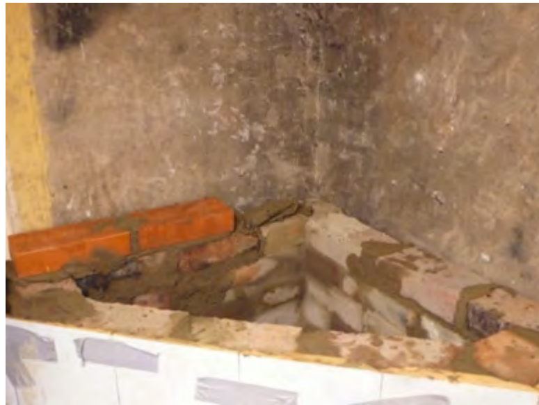
Figure 2.51. When we reached the top of tile row 7, we ran out of old bricks and started to use new PT-standard bricks.
