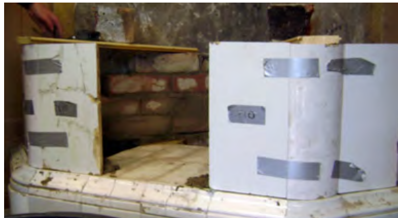
Figure 2.27. Our first row of tiles, marked number 10, is in place. Tape is used to hold the tiles until the mortar has set.
