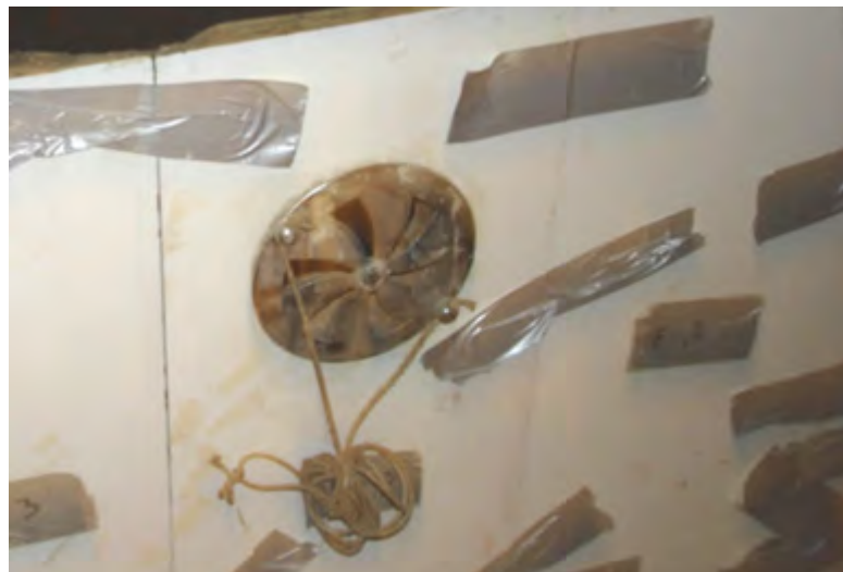
Figure 1.45. Rosette air vent in the last row of tiles before installing cornice.
