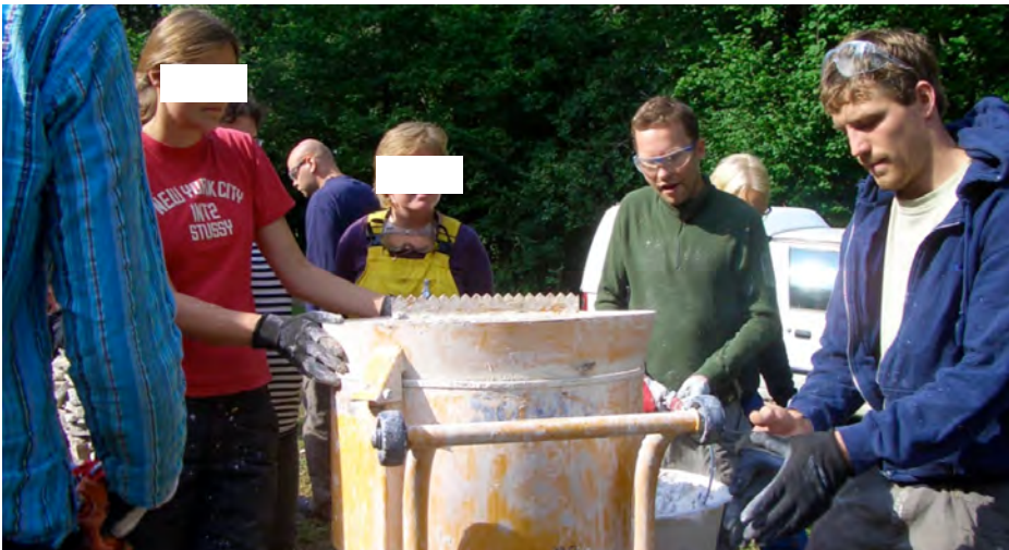
Figure 12. Making bigger quantities of lime render by using a roller pan mortar mill.
